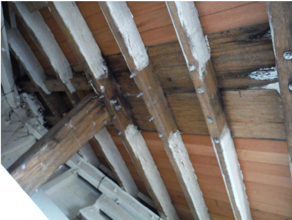
VIEW OF UNDERSIDE OF KING PLANK 6 WHITE & BLACK AREA IS ROT
